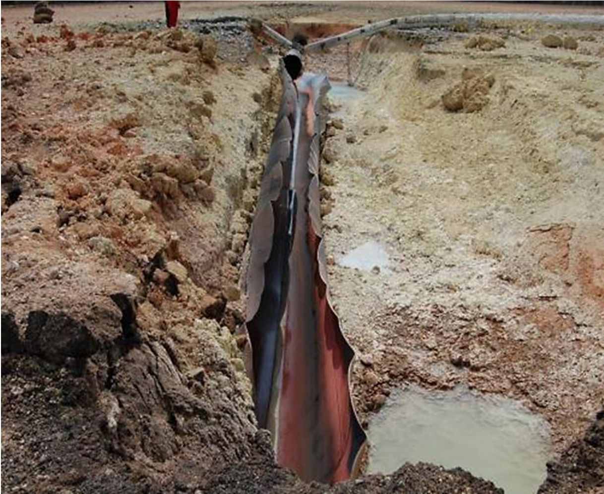
Figure 3. Ruptured section, about 110 feet long, of 36-inch-diameter Enterprise natural gas pipeline
