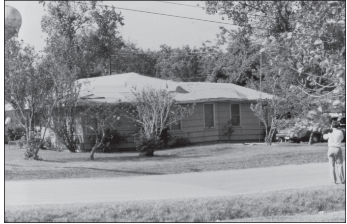
Figure 10. House wracked by surface faulting in Baytown, Texas, near Houston. Faulting here is manifested by flexure of land surface. Photograph by Thomas L. Holzer, October 1983.
